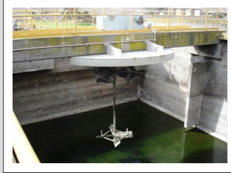
Large Aerator Paddles place huge pressure on gearboxes, motors and lubricant.
