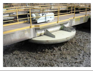
Aerator gearboxes working under full load
